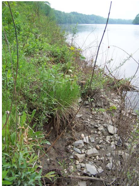
Localized Erosion between survey stakes 34 and 35. Looking upstream May 2006
