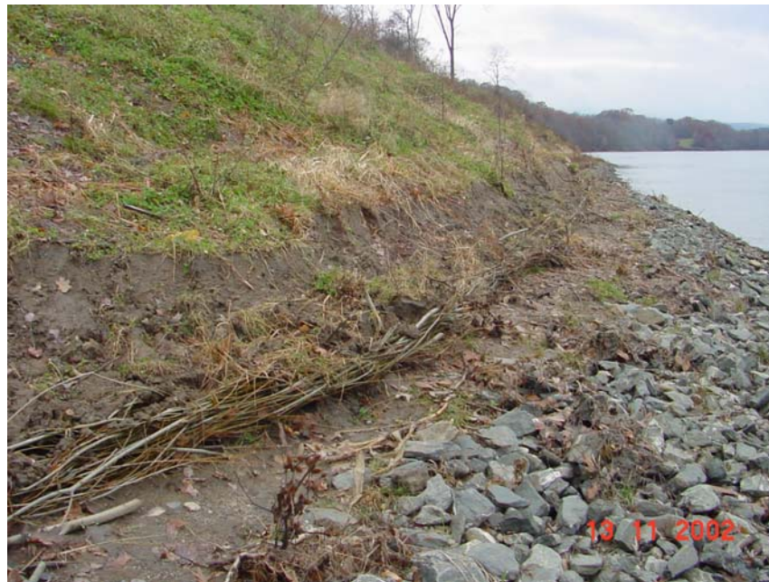
Installation of Coir Fascines and Live Stakes at Urgiel Upstream Site November 2002
