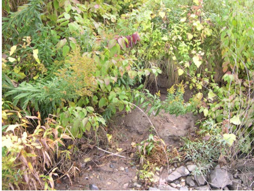
Localized Erosion at Stone Toe/Lower Slope Interface at the Urgiel Upstream site between survey stakes 34 and 35– October 2006
