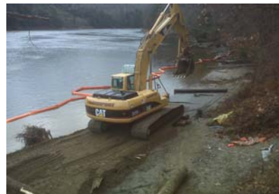
View of the construction of the last 100 feet of the aquatic bench.
