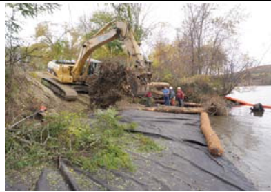
View of the start of construction on the root wads structures and bench.
