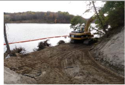
View from access ramp of construction of the root wad structures and bench.
