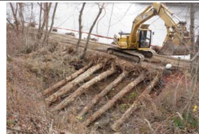
View of LWD within the scalloped eroded areas.
