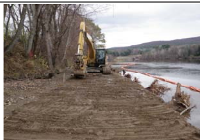
View the operator "dressing out" or stabilizing the bench. This is performed each night before the crews leave the site.
