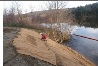
View of the start of the restoration treatment to the access road.
